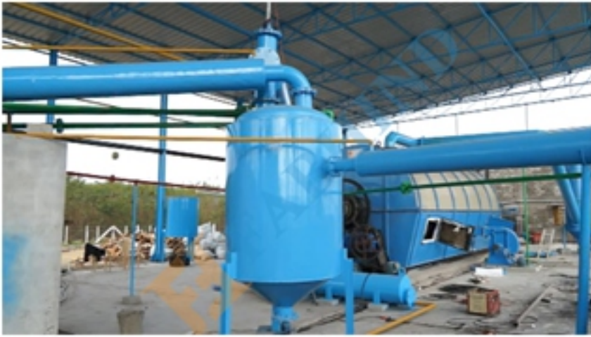
Water Seal Tank
